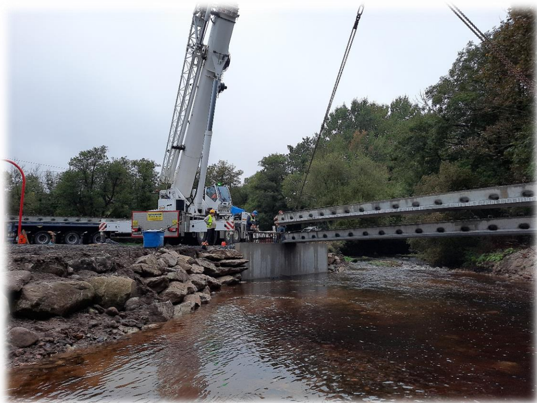
Figure 3.8 Brooklodge bridge, Borris, Co. Carlow under reconstruction to prevent restrictions causing flooding upstream.
