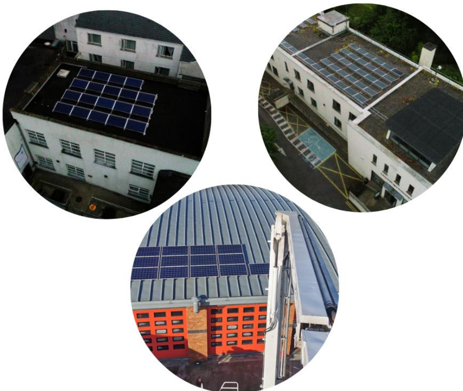
Figure 3.12 Solar PVs in Use on Carlow County Council Buildings.
